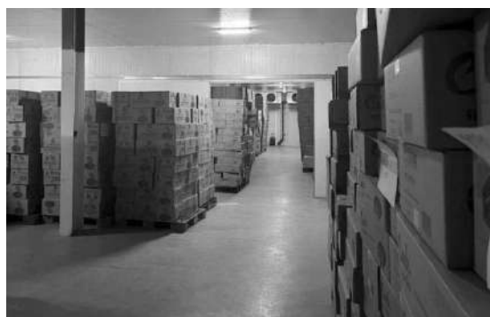
Our chiller room in Building 1
